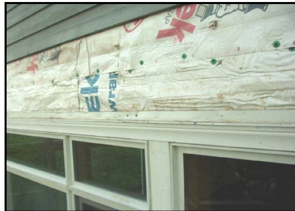
Windows (incorrectly) have flange over house wrap
