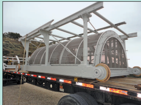
Newly refurbished intake gate assembly arriving ready to be returned to service.
