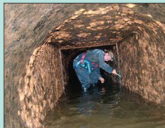
Scott MacDonald performing maintenance on 4'x4' emergency gate guides deep inside dam's outlet works.
